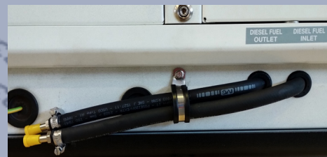
INPUT/OUTPUT FUEL PIPE
