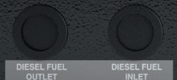
INPUT/OUTPUT FUEL PIPE
