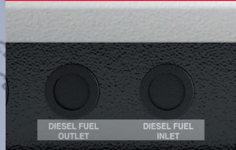
INPUT/OUTPUT FUEL PIPE
